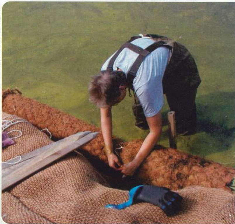
Protection for newly planted vegetation is critical, or wave action and surface runoff will uproot the plants before they can establish. Here, Carolyn Dindorf of Fortin Consulting works with a coir roll and erosion control fabric.
